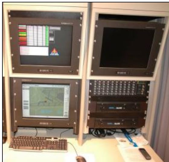
Figure 10. IOS Station Inside COVE Lab Trailer
